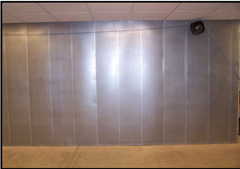
Figure 3.1 Supplied Air Wall. Air movement designed to force air contaminants down range away from instructors and shooters.
