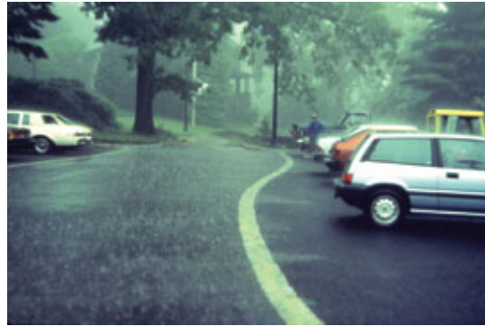
Figure 15: Example Porous Pavement Application (Adams, 2003). Water pools on the conventional asphalt on the left, but is able to infiltrate the porous asphalt on the right.
