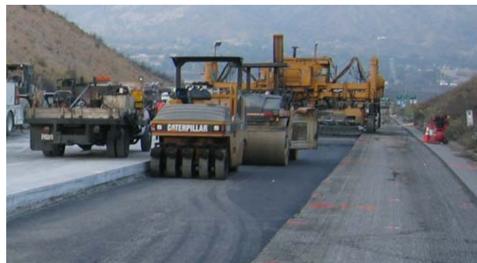
Figure 6: HMA Application (CA DOT, 2006). After HMA is laid, it is then rolled to produce a dense, smooth surface.
