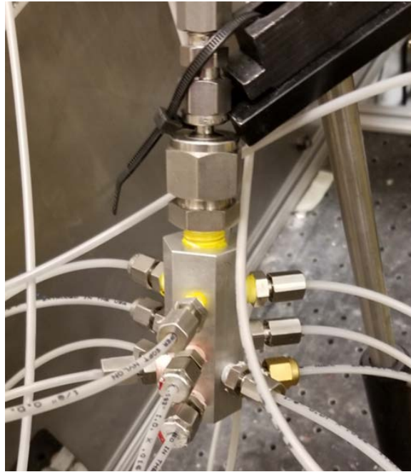
Figure 30. The propane manifold used to fuel the new combustor fed by the Alicat controller.
