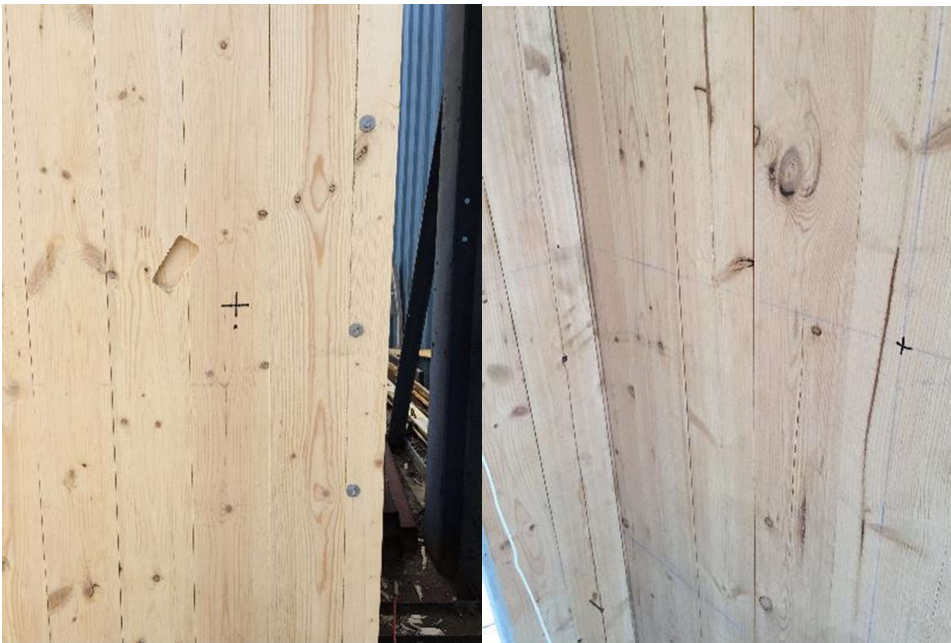
Figure A-17: Panel 6, weak-axis, strong-connection, edge, 12-pound, 77.6 mph, passed (front-left, back-right)
