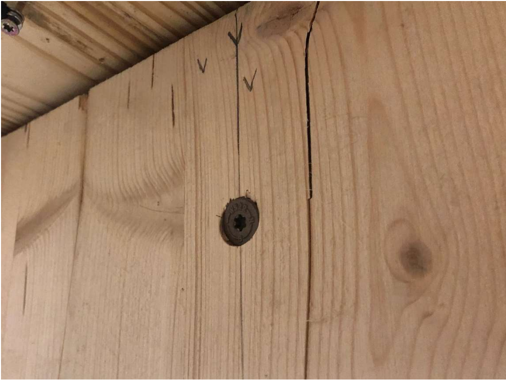
Figure 4.36: Deformations in connection between in-plane and out-of-plane walls
