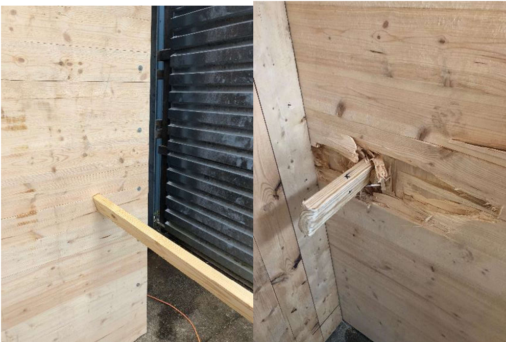
Figure A-35: Panel 12, strong-axis, strong-connection, edge, 14.5-pound, 105.8 mph, failed – perforation/dislodgement (front-left, back-right)
