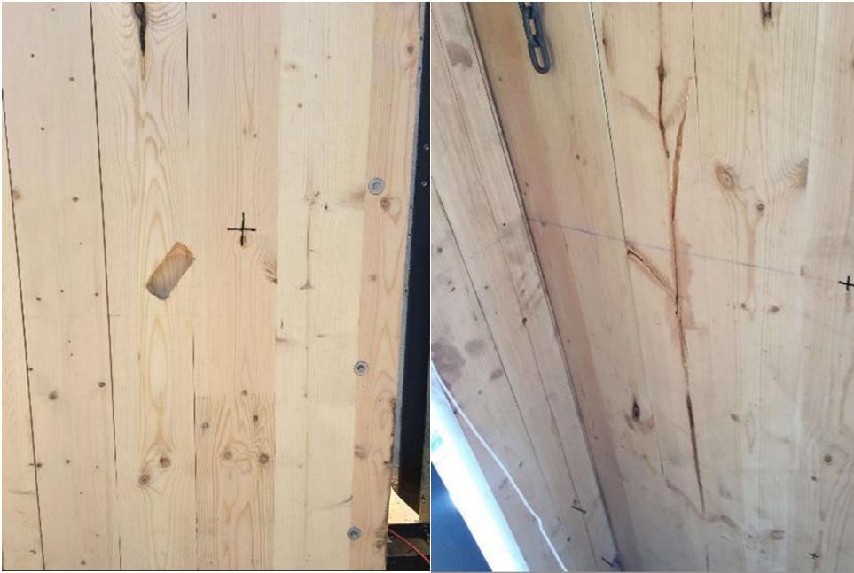
Figure A-14: Panel 5, weak-axis, strong-connection, edge, 15-pound, 88.1 mph, passed (front-left, back-right)
