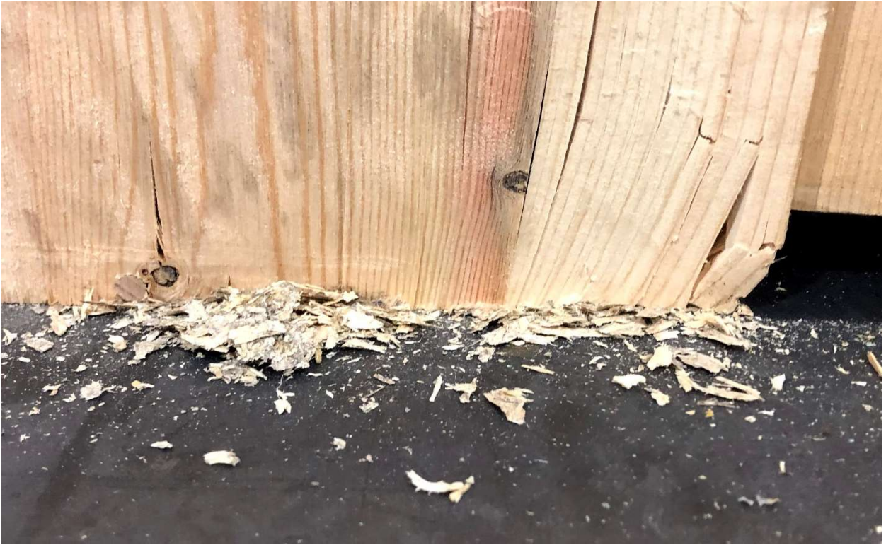
Figure 4.37: Crushing of wood at half-lap joint between in-plane wall
