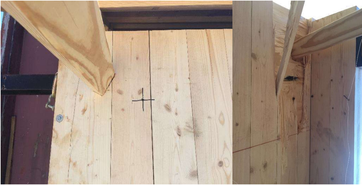
Figure A-12: Panel 4, weak-axis, strong-connection, corner, 12-pound, 102.4 mph, failed – perforation (front-left, back-right)
