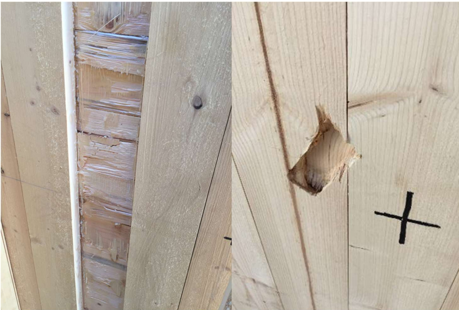
Figure A-5: Panel 2, weak-axis, strong-connection, edge, 15-pound, 84.1 mph, failed test – dislodgement (back-left, front-right)
