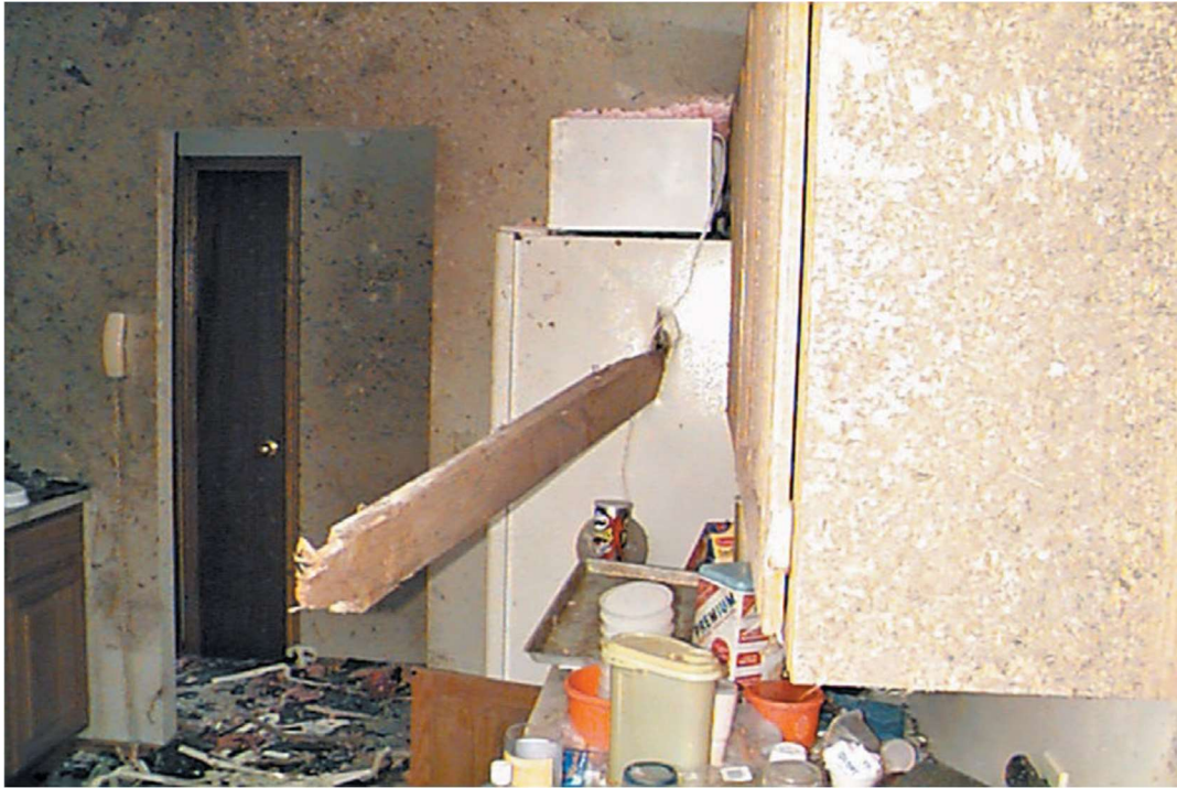
Figure 2.2: Windborne debris damage from a 2x6 framing element
