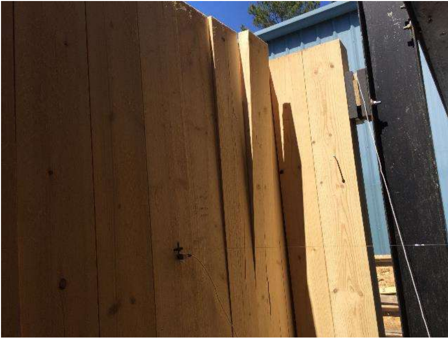
Figure A-6: Panel 2, weak-axis, strong-connection, corner, 15-pound, 80.9 mph, passed test (back of panel)
