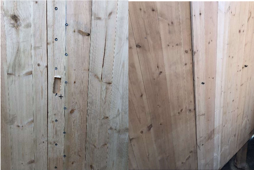
Figure A-44: Panel 16, weak-axis, half-lap connection, center, 15-pound, 68.5 mph, passed (front-left, back-right)
