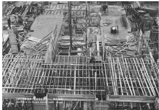
Figure 2. Velasca tower, Milan. Construction of a typical floor (Italian State Central Archive, SGI-Sogene Fonds, Rome).
