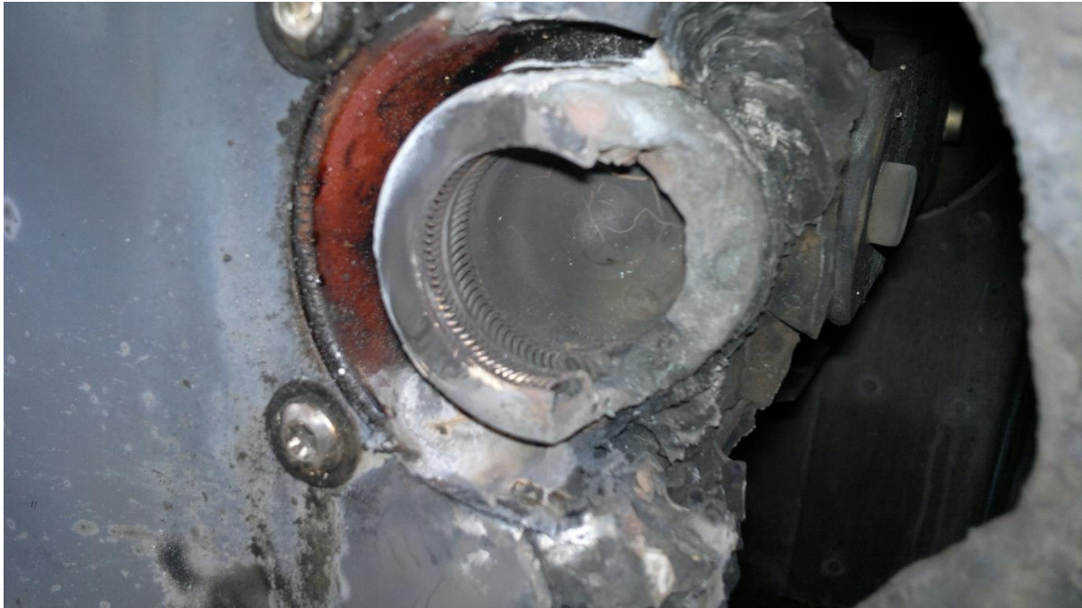
Fig. 1. Consequences of earth connection and 22 kV non-fired arc.
