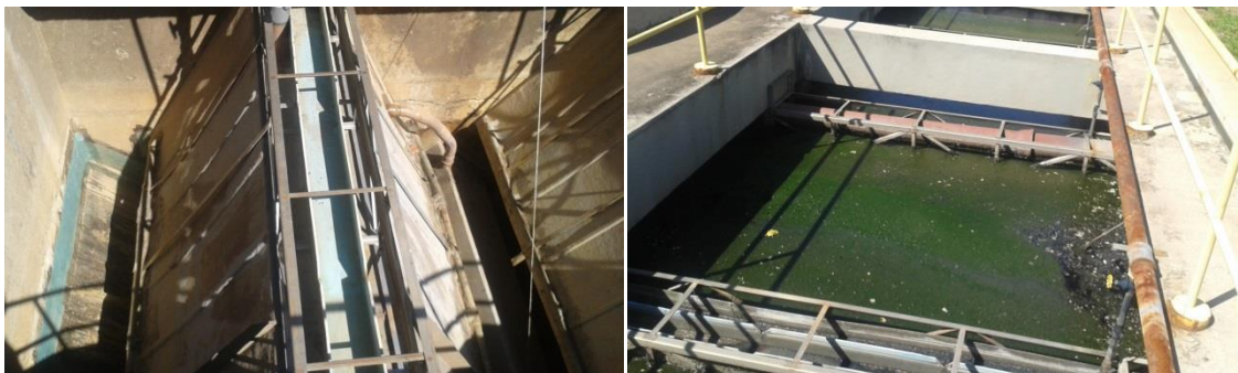
Figura 1 - Reator UASB vazio. Figure 1 - Empty UASB reactor.
