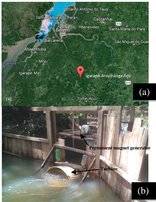
Figure 1. (a) Location of the creek; (b) Hydrokinetic turbine installed at Arapiranga-Açu.
