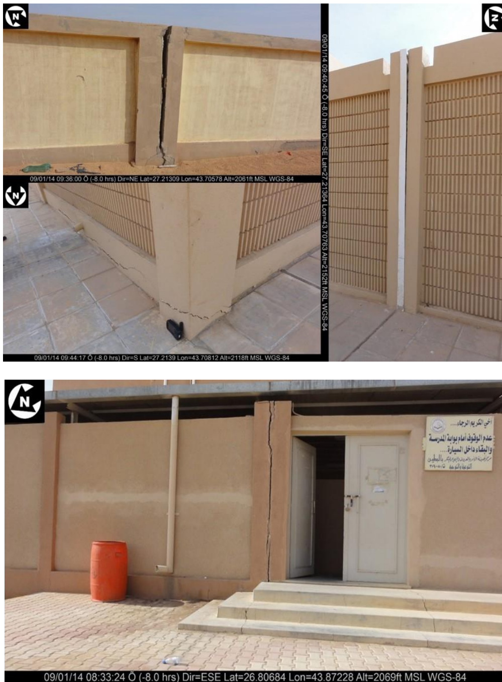
Figure 3.2 Big cracks on wall school buildings at the Mudarraaj city areas.
