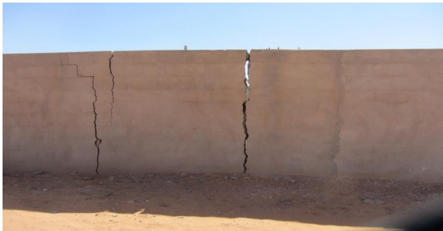
Figure 3.1 Cracks on wall house buildings at the Turubah city areas.
