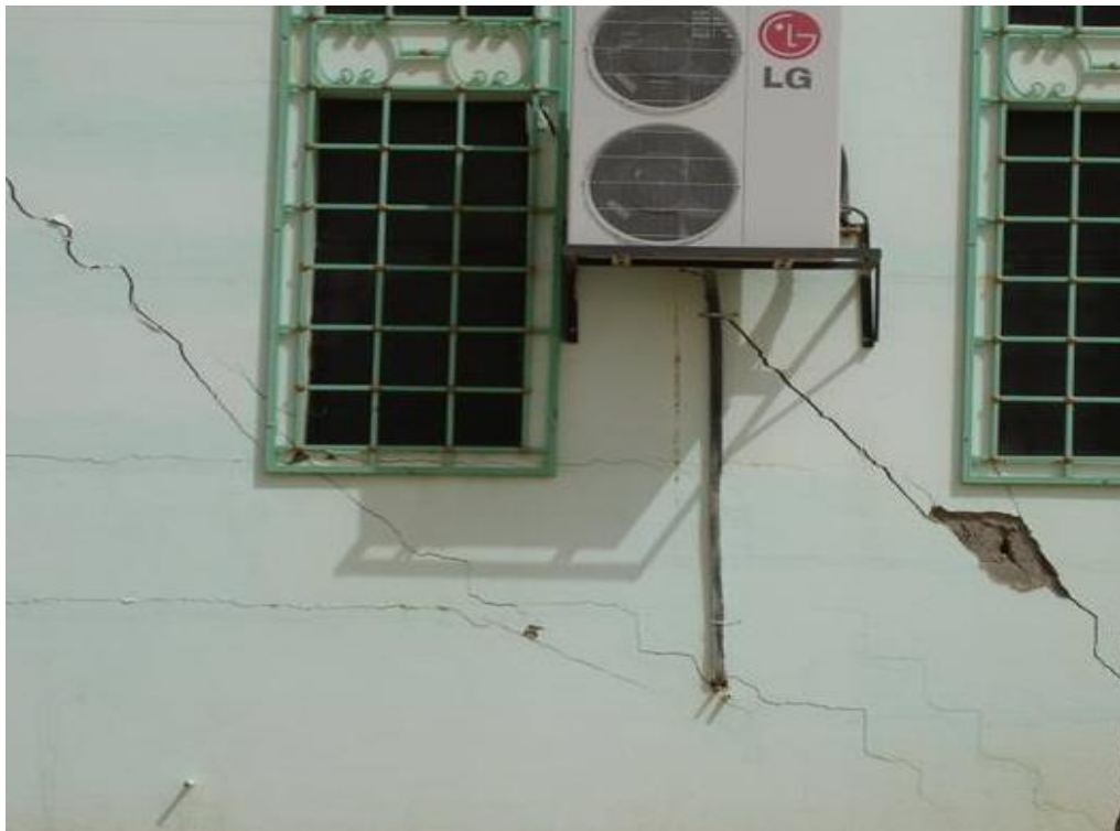
Figure 3.3 Big cracks on buildings at the Mudarraaj city areas.
