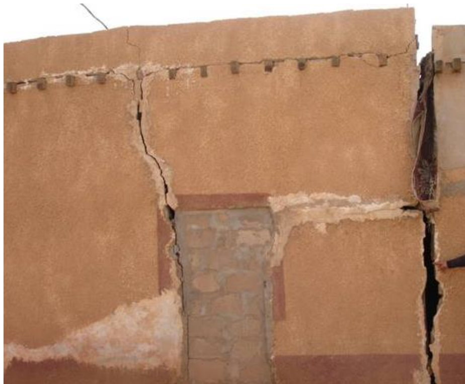
Figure 3.4 Significant cracks on buildings at the AL Butayn city areas.
