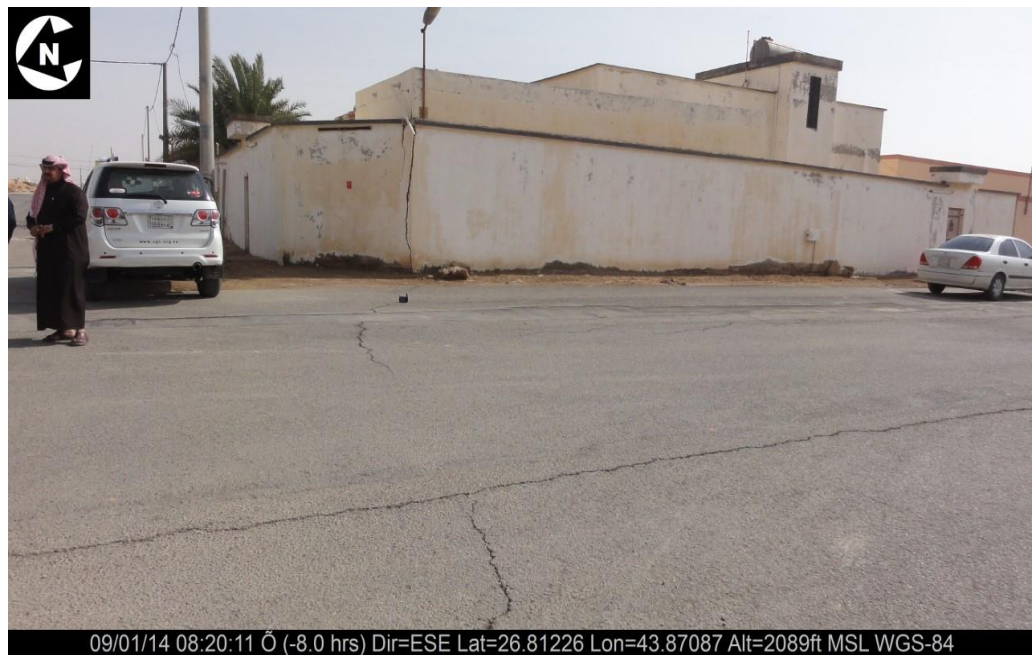
Figure 3.8 Some types of cracks on buildings and street at the AL Butayn city areas.
