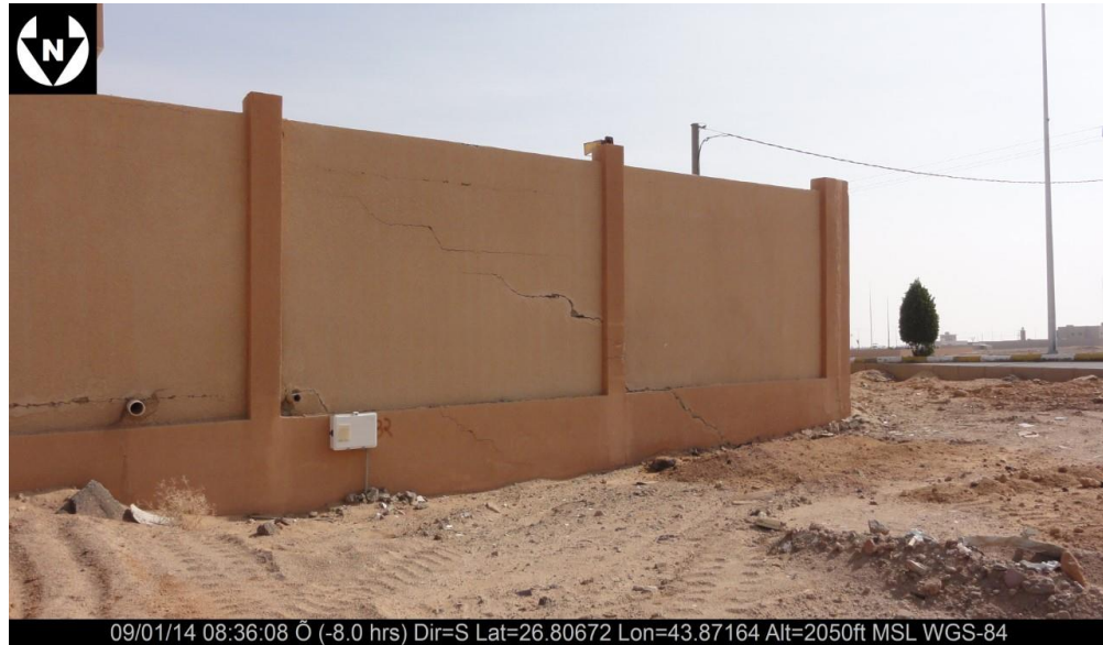
Figure 3.9 Some types of cracks on buildings and street at the studies areas.
