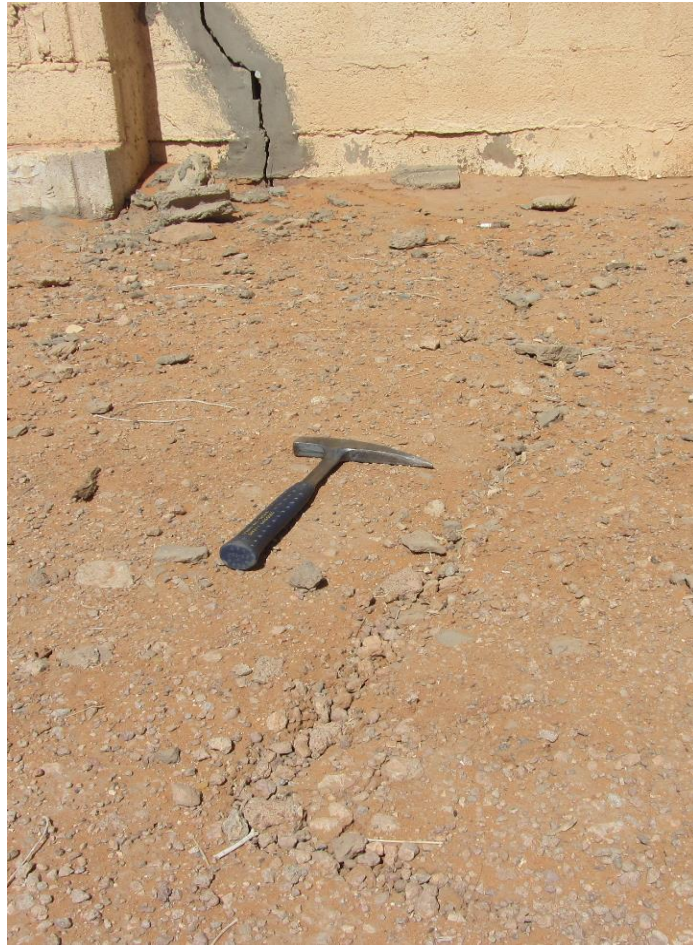
Figure 3.5 Some types of cracks and fissure at the studies areas.
