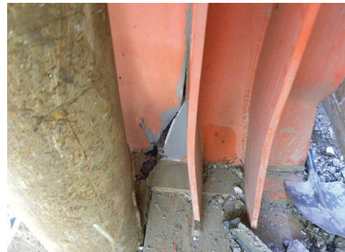
Fig. 3. Girder fracture at the NE abutment
