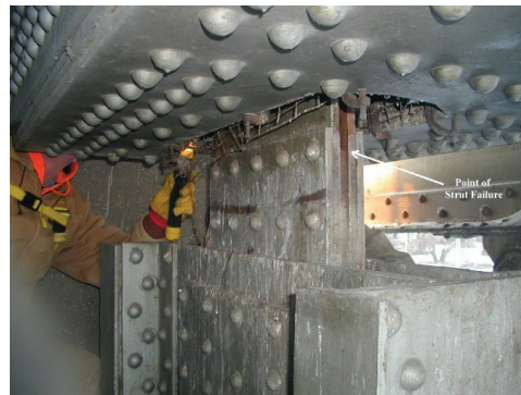
Fig. 2. Point of strut failure
