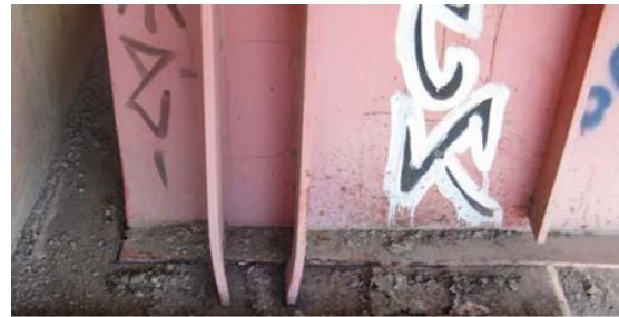
Fig. 2. Fillet weld fracture of the girder-to-masonry plate connection at the SW abutment
