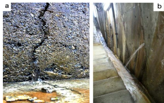
Fig. 4. Visual inspection results: a- a crack with water pouring through, b- water filtration inside the dam
