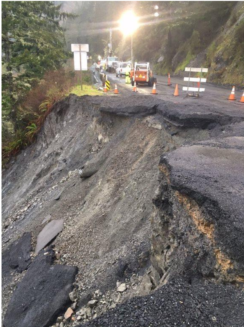
FIGURE 2-3: LAST CHANCE GRADE SLIDE
