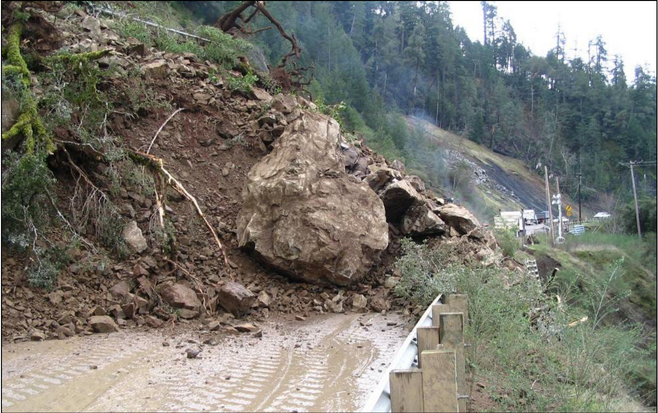
Figure 11-7. Confusion Hill Slide, View Looking South on U.S. Highway 101, Winter 2005-06
