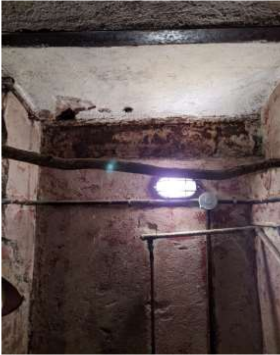
Figure 10 Oxidation of metal supports, author photo.
