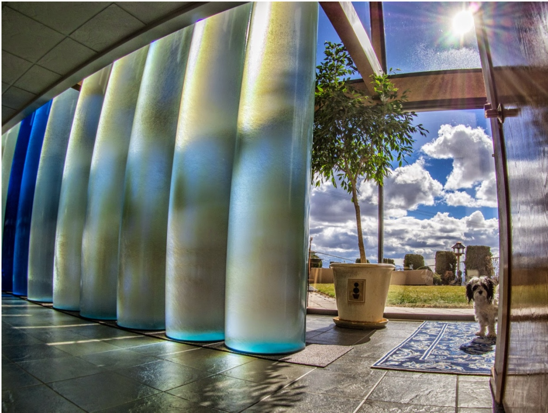
Figure 4. Solar storage water tubes.
