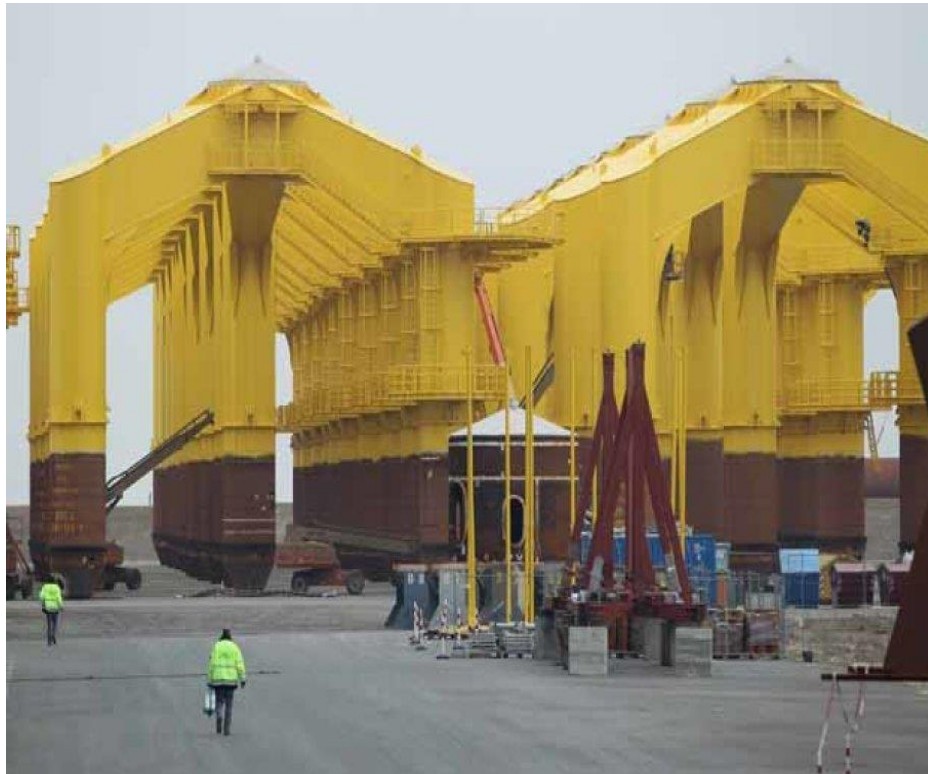
Figure 101 The massive three-pronged steel legs, required for the anchoring to the sea bed 108
