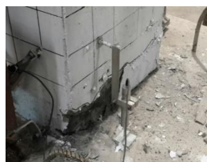
(c) Crack at the column base
