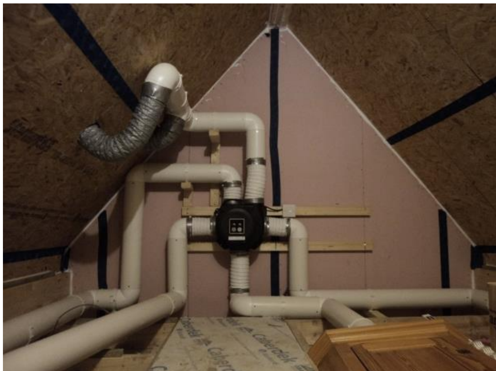
Fig. 5.17 UK54's mechanical ventilation system MEV (no heat recovery)
