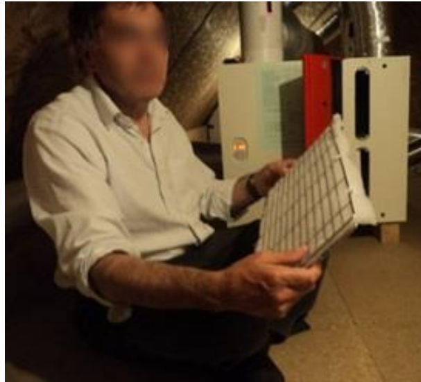
Fig. 5.22 Occupant showing to the researcher the filter component of the MVHR system
