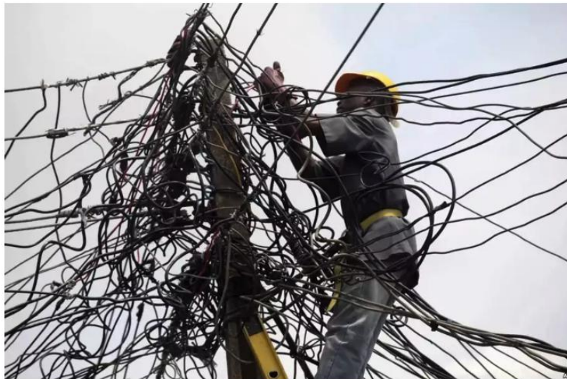
Figure 1: Sample of a distribution line that are not properly maintained
