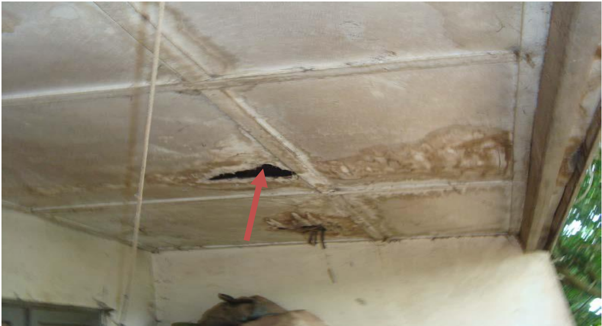
Figure 3f: Plate 6: Damaged Ceiling of one of the classroom blocks at Wa Islamic Girls Senior High School
