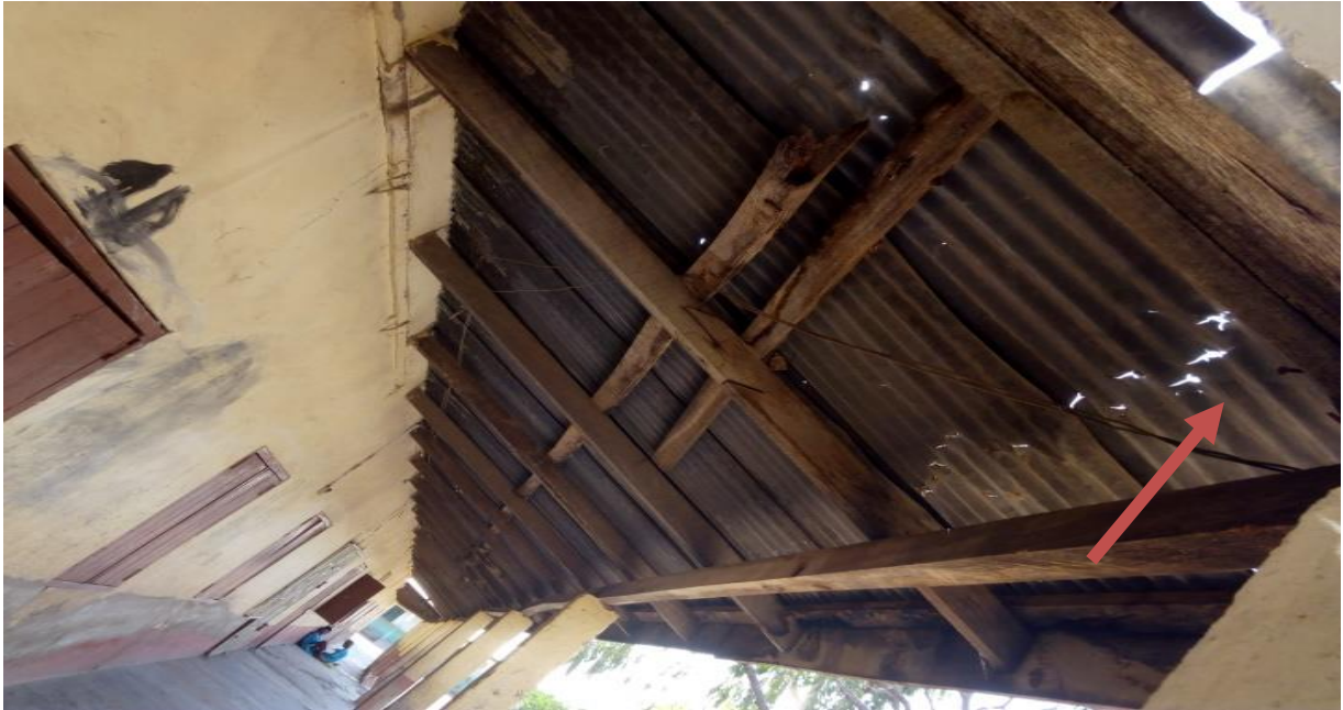
Figure 3a: Damaged Classroom Roof at Wa Islamic Girls SHS
