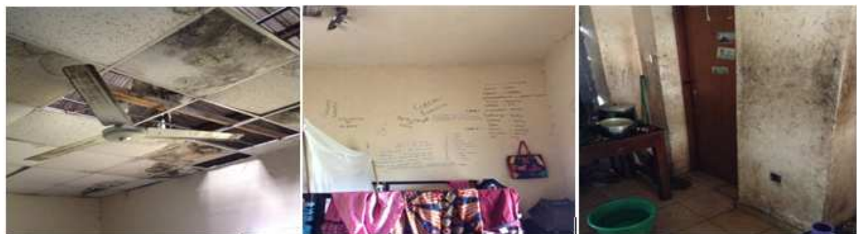
(j) Unsuitable ceiling
