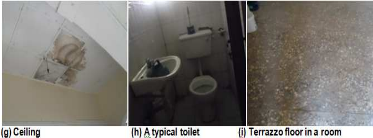
Figure 5.43 Photos showing conditions of some facilities in the chalets
