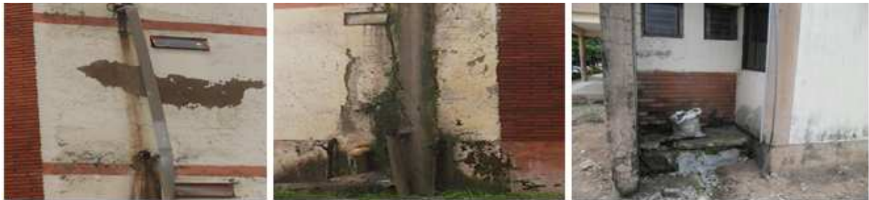
Figure 5.18 Deteriorated plumbing services at the hostels at Case A3
