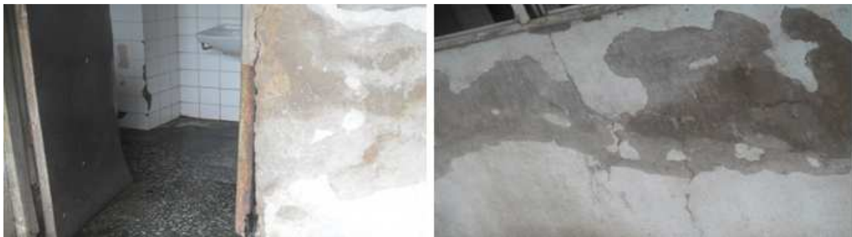
Figure 5.12 Decaying wall and door of a bathroom at Case A2
