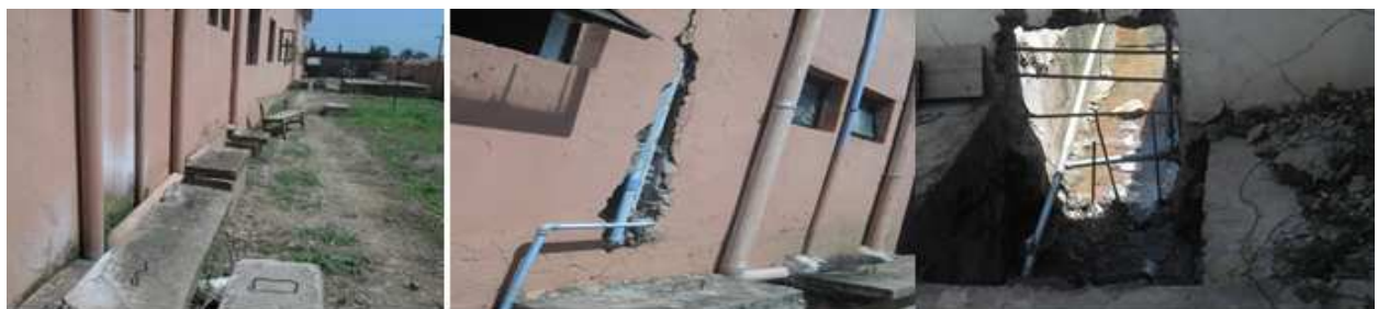
Figure 5. 60 Plumbing conditions around the hostels at Case C3
