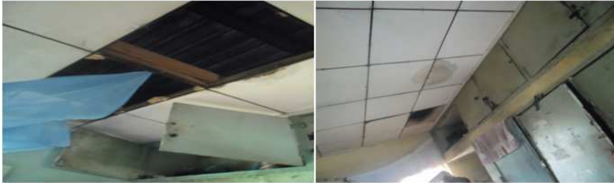
Figure 5.13 Dilapidated ceilings in some of the rooms at a hostel block at Case A2
