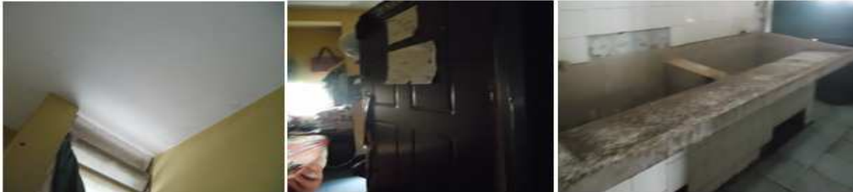
(g) Ceiling and wall of a room (h) Bedroom (i) Laundry
