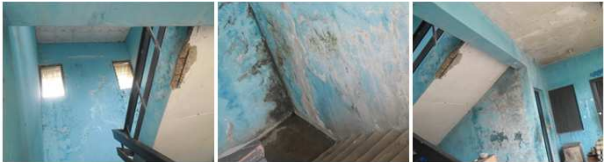
Figure 5.25 Poor condition of a stair well at Case B1
