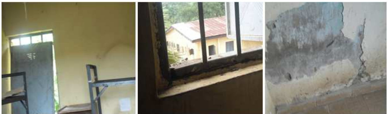
Figure 5.26 Samples of unsuitable conditions of windows and wall in a bedroom at Case B1
