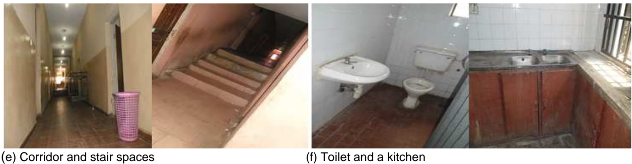
Figure 5. 59 Photos showing condition of components within hostels at Case C3
