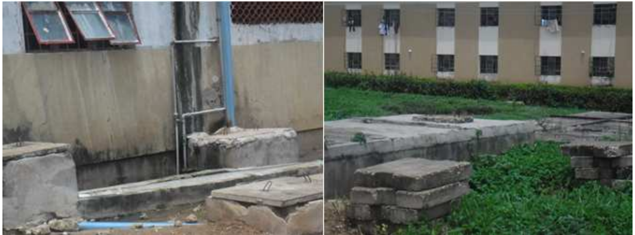
Figure 5.10 Poor conditions of inspection chambers and soakaways behind hostels at Case A2
