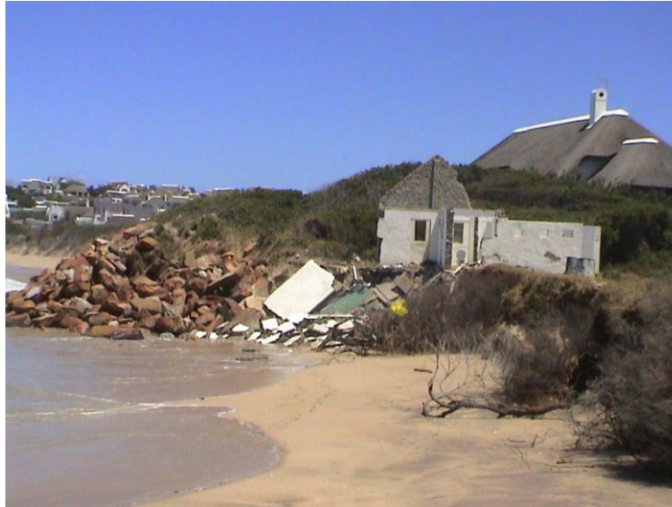
Figure 2.40 Erosion in November 2005 began undermining the public toilets at Anne Avenue and the storm waves in August and September 2006 resulted in the total collapse of this structure (picture by Illenberger).
