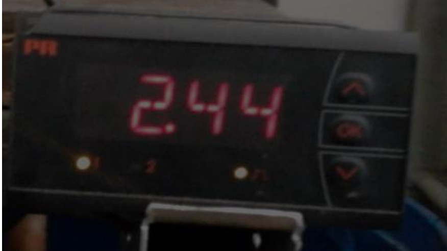
Figure 3.11 Picture of a flow meter for working fluid
