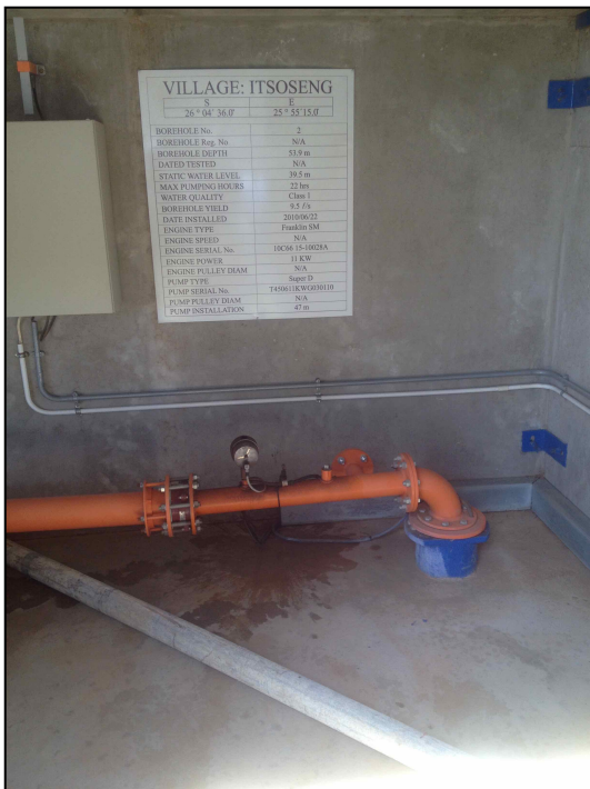
Public water supply borehole at Itsoseng, in the south of the Grootfontein aquifer.
