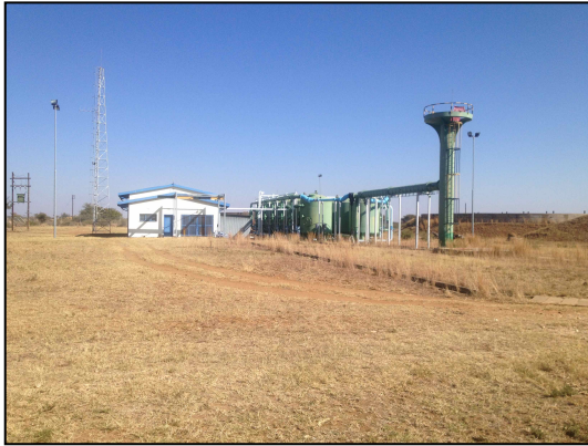
The Mafikeng Water Treatment Works, which receives water from the Molopo Eye and the Grootfontein boreholes.
