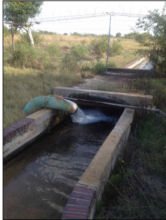
Grootfontein boreholes discharge into a concrete channel. The water is then piped to the Mafikeng Water Treatment Plant.
