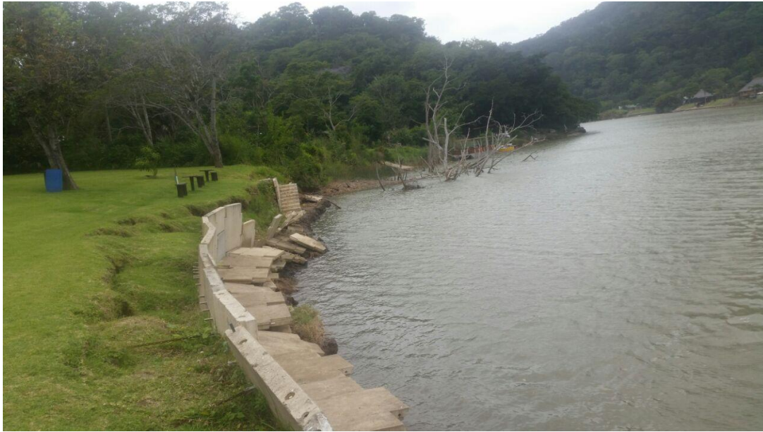
Figure 6.12: Concrete walls used as a preventive measure against floods.
