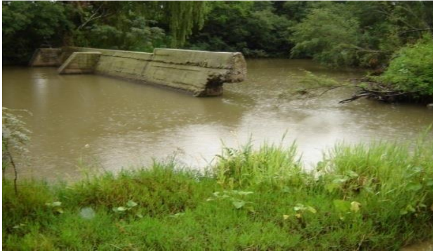
Fig. 2.9 Study Site 8: Honeydale (32° 48' 157" S, 26° 51' 607" E) showing typical characteristics of good availability of a wide range of macroinvertebrate biotopes
