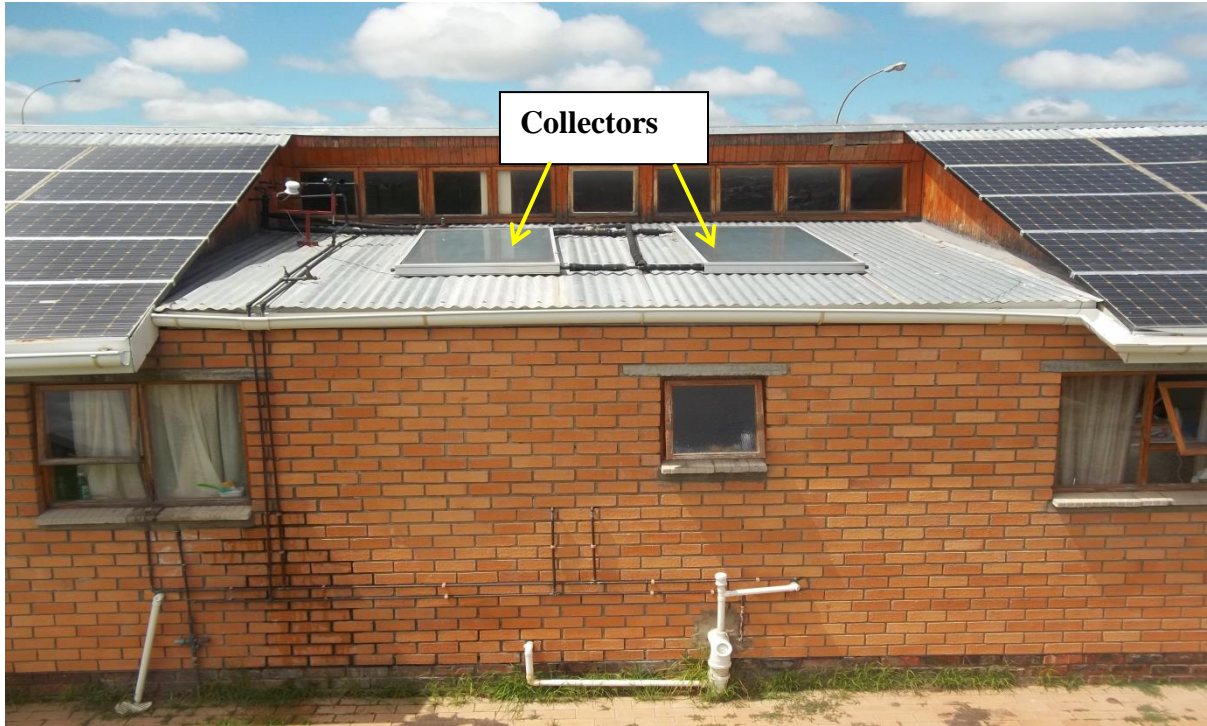
Figure 3.1: Solar House University of Fort Hare. Roof showing solar collector panels.
