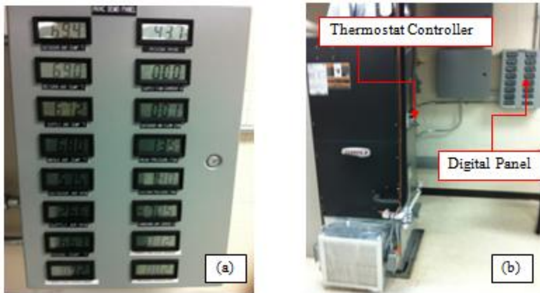
Figure 10. (a) Digital Panel, (b) Digital Panel connected to the system controllers
