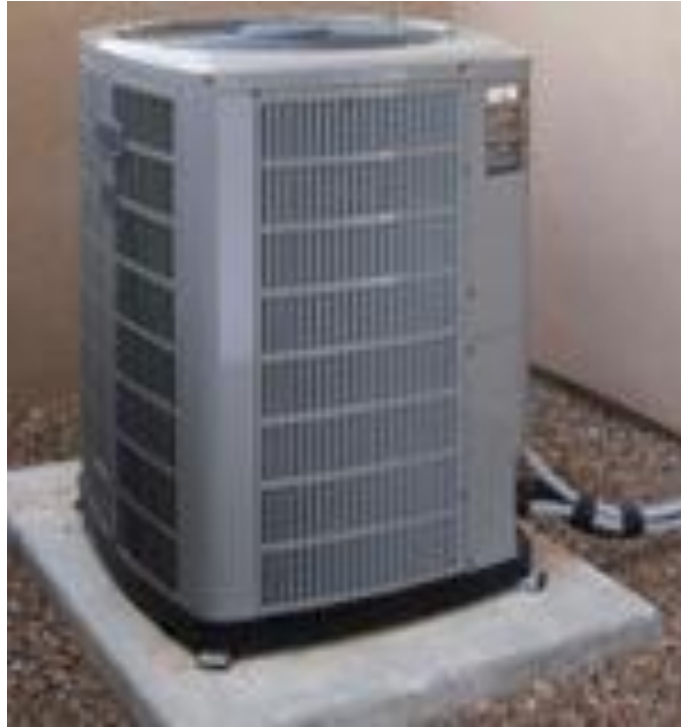
Figure 8. The condenser/compressor unit of typical residential split-system heat pump.
