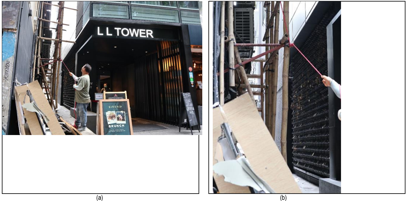
Fig. 3. (a) An outdoor VGS was built on a façade facing a narrow alley between two tall buildings. (b) A close up view showing dead wilted plants remains on this VGS.
