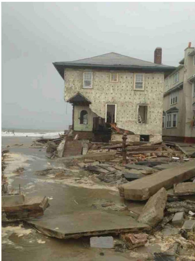
Figure 1.5. House on Brooklyn shorefront after Sandy. Photo by “Proud Novice,” 2012. ( https://commons.wikimedia.org/wiki/File:Damage_from_Hurricane_Sandy_to_house_in_Brooklyn,_NY.jpeg ). Creative Commons License BY-SA 3.0.
