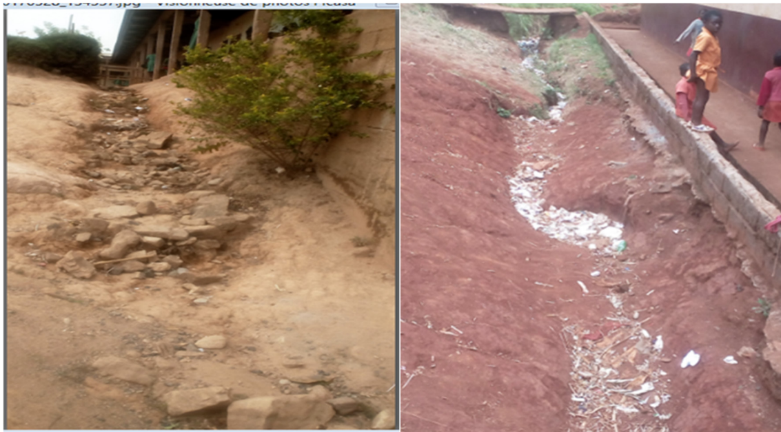
Figure 12. Absence or poor condition of the channels
