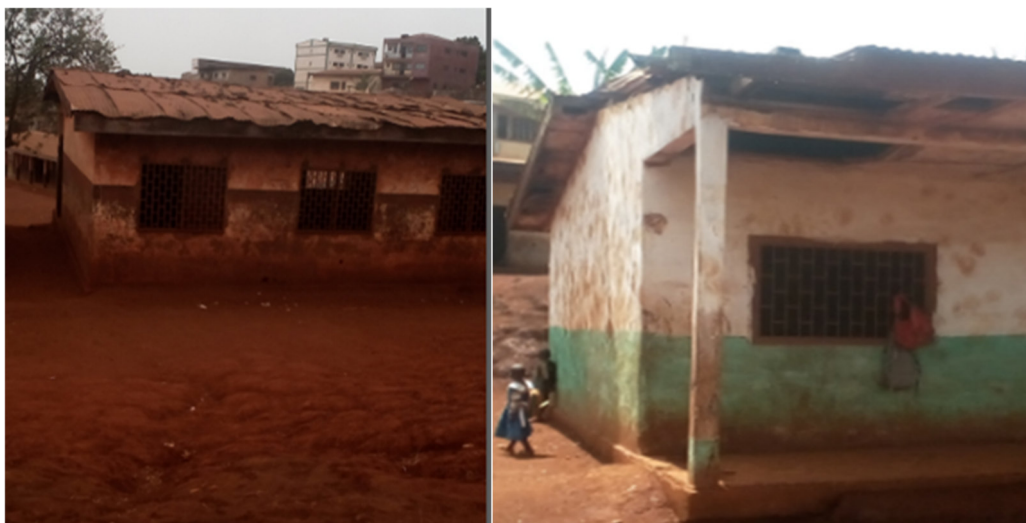
Figure 16. Poor paint condition / paint aging
