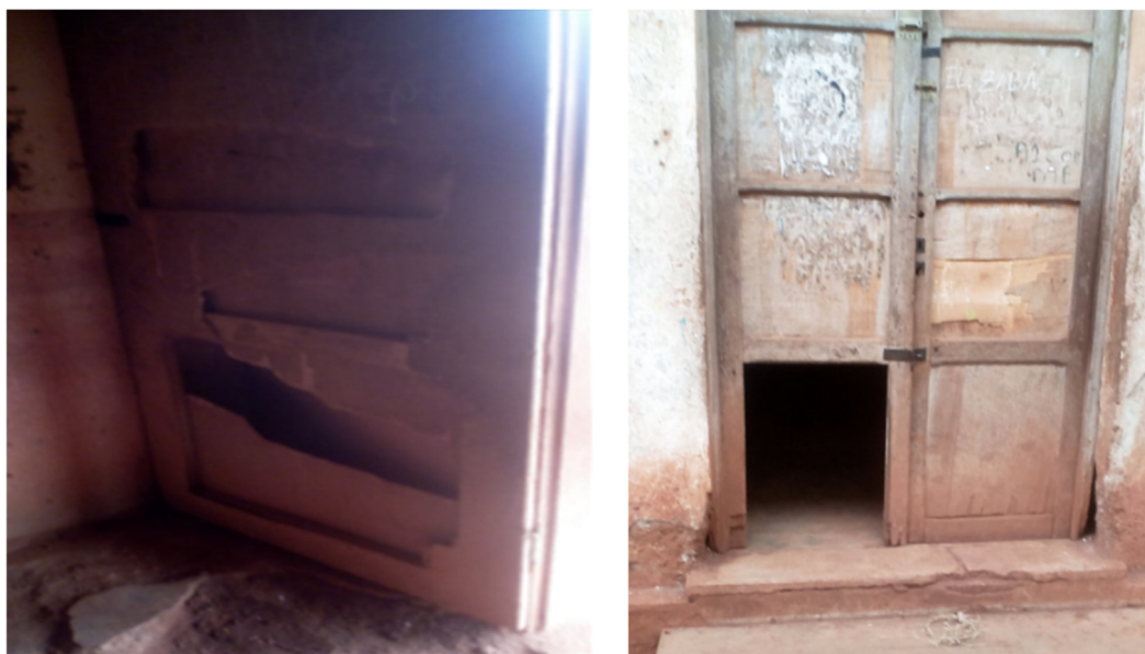
Figure 4. Poor condition of the doors of some school buildings
