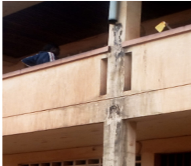
Figure 9. Defective water descent
