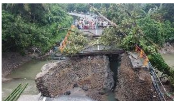
Figure 1. Condition of Batang Kalu Bridge damage caused by massive toe scouring occurred due to increasing flow at the bottom.
