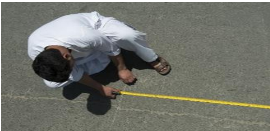
Fig. 3: Transverse crack in flexible Pavement [24].
