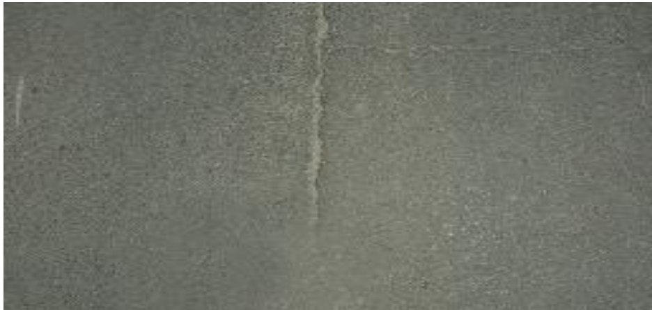
Fig. 2: Longitudinal crack in flexible Pavement
