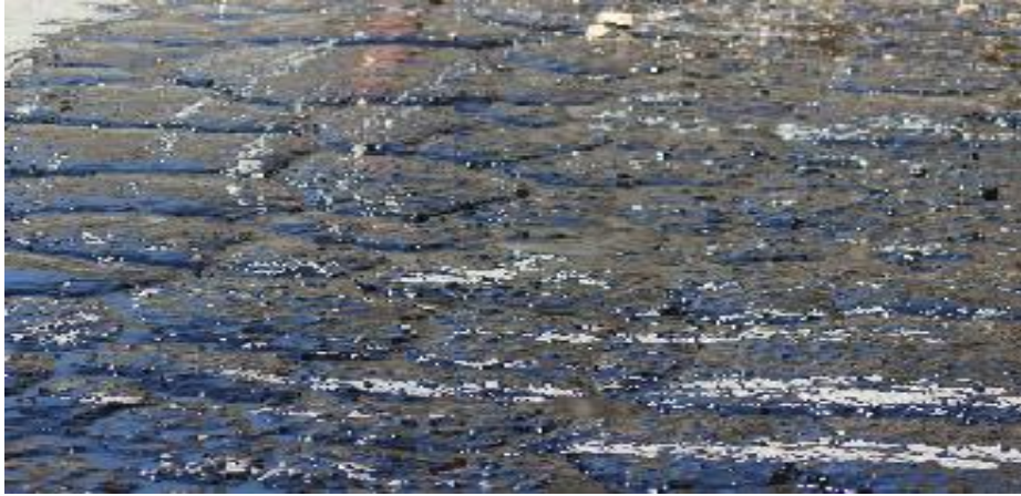
Fig. 1: Crocodile Cracks in flexible Pavement
