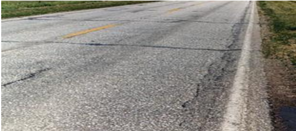
Fig.6: Rutting crack in flexible Pavement
