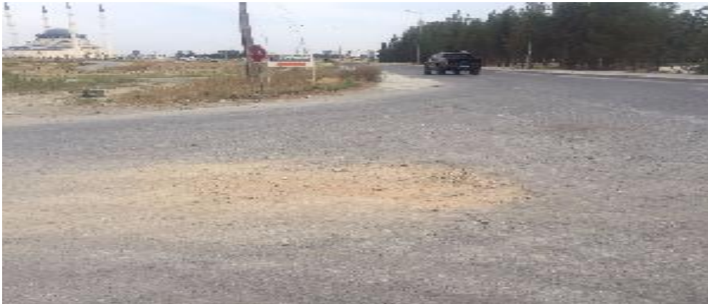
Fig.7: Pothole in flexible Pavement
