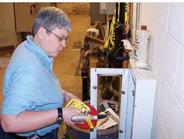
▲ Dawn Harrington, 76, on the job – checking safety systems at Independence National Historical Park.
