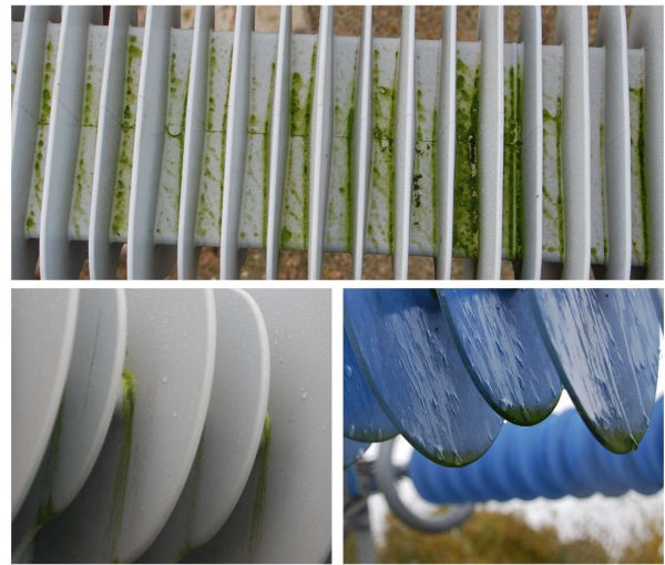
Figure 11. Top: Aerial photo of growth of algae in the central region of the compression element SCc after 35 months in service. Bottom left: the run-off of water from the top horizontal surface down the vertical shed led to a spread of algae. Bottom right: The tension insulator STc can be seen to have accumulated algae on the bottom of the sheds, and also to have lost much of its hydrophobicity.
