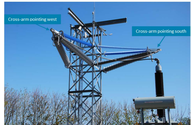
Figure 2. Photograph of the trial site, showing two cross-arms and the high voltage bushing. The cross-arm on the right points due south (along the coastline) and the other points west (away from the coastline).
