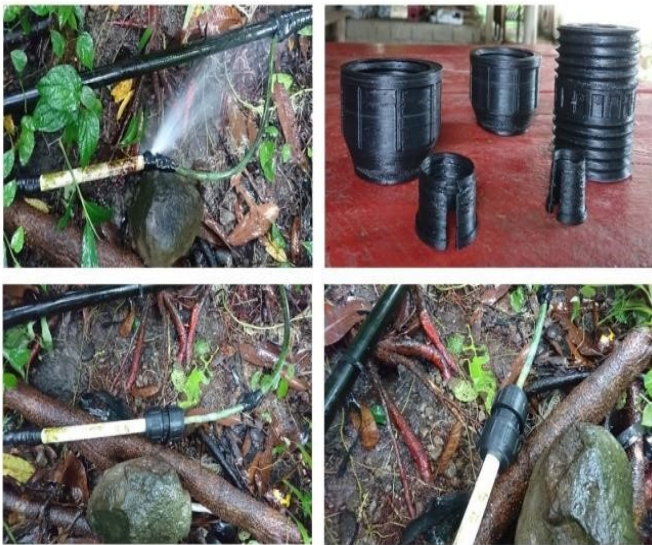
Fig. 7. Leaking and fixed water pipe and the 3D printed pipe connector made from recycled plastic
