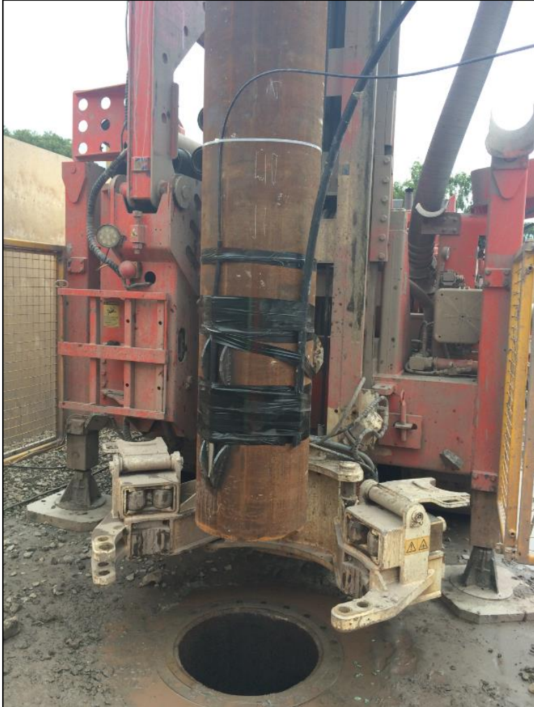
Figure 5 Photograph of the bottom section of the steel superficial deposits casing with fibre-optic cable attached and welded centraliser, during installation at GGA02 on 18/07/2019
