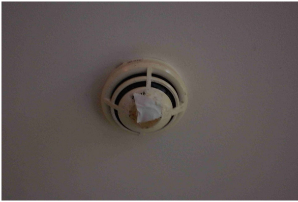
Fig. 4 Masking tape on smoke detector
