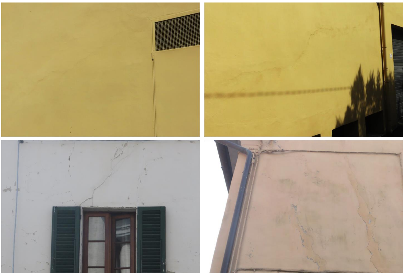
Figure 35 – Cracks evidence in Pistoia historical center buildings.
