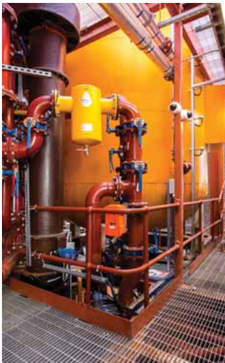
An interior shot of the Bunhill 2 Energy Centre on the edge of City Road, Islington.
