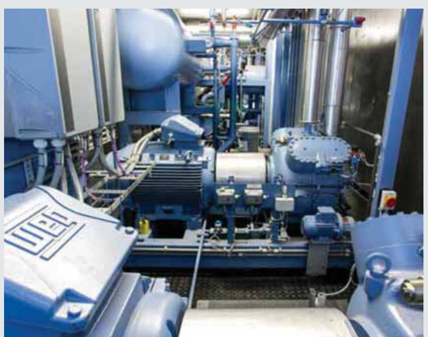
The heat pump in the new energy centre.
