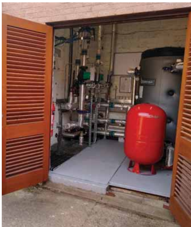
Hidros LHA feeds into a Cordivari multi-connection insulated buffer tank with a back-up high-efficiency gas-fired boiler.
