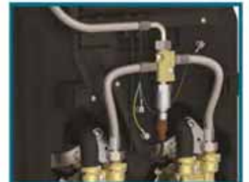
Pressure Transducer Control
