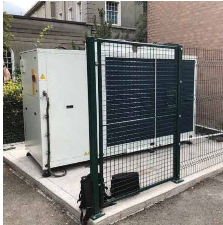
The Hidros unit was delivered and located on a pre-formed concrete plinth for ease of handling and installation simplicity.
