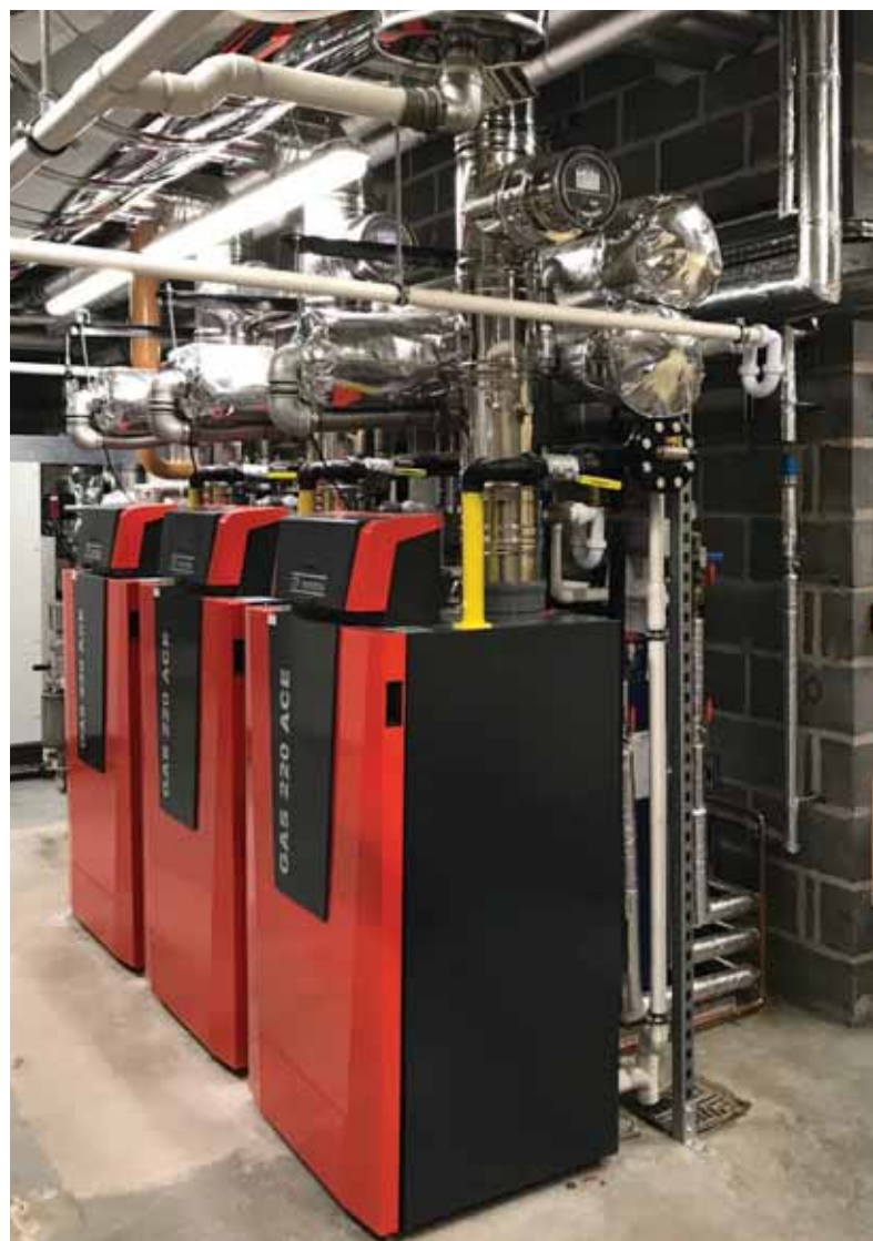
The ability of modern boilers to be installed in modular configuration enables large outputs to be installed in a tiny footprint, as well as in hard-to-reach areas.
