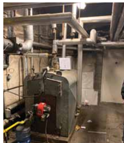
Before – Plantroom prior to work commencement.
