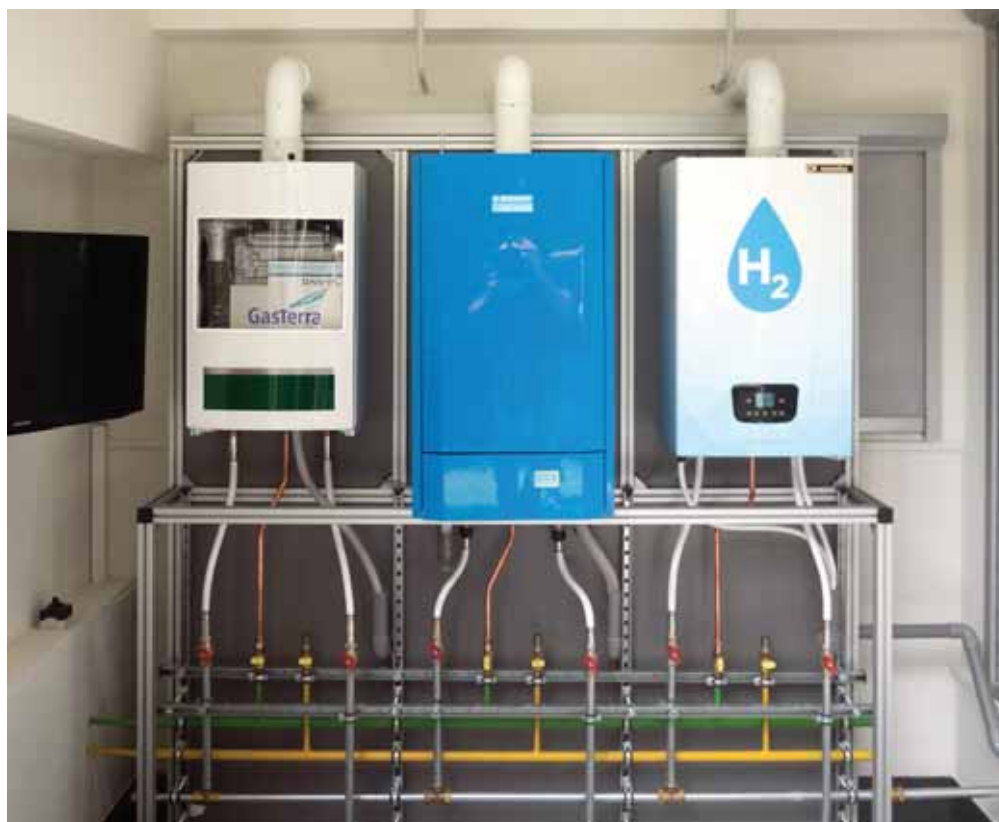
Image of the plant room with the hydrogen boiler in position next to the conventional natural gas boilers at the housing cooperative project in Rozenburg, the Netherlands.
