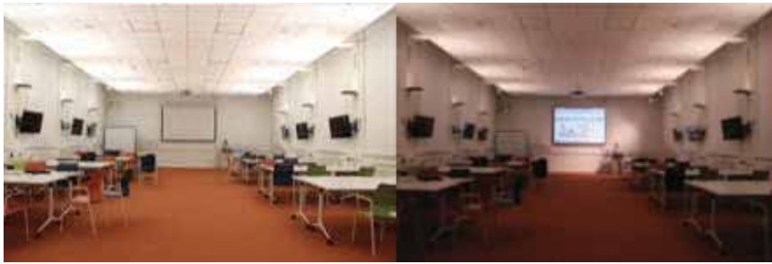
Figure 7 – Updated lighting using TAIR, full output on left and dimmed on right.
