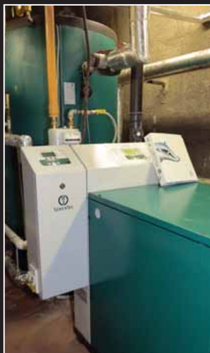
The SenerTec Dachs CHP.
