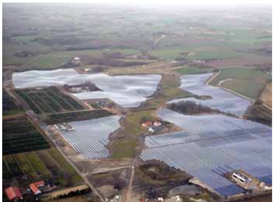
Figure 3: Solar thermal district heating plant in Silkeborg, Denmark [5] .
