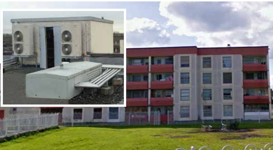
DI Big (RAVSM2804AT8) units are installed on all eight blocks.
