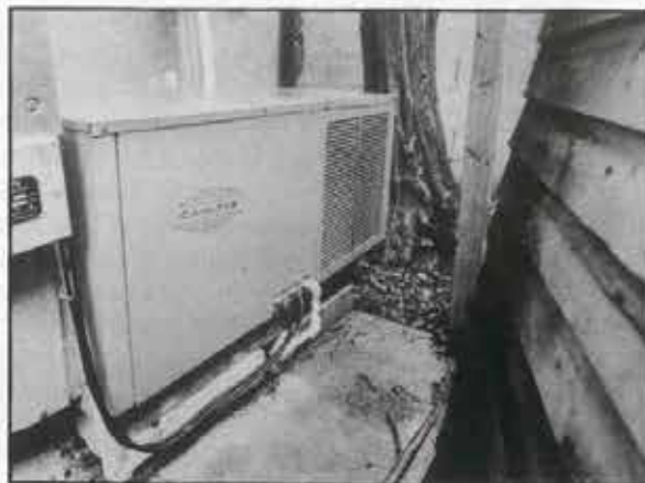
● Picture shows the Carlyle 50DQ024 packaged heat pump installed at John Freestone's house, in Dublin.
