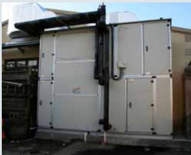
Heat recovery LTHW pool unit.
