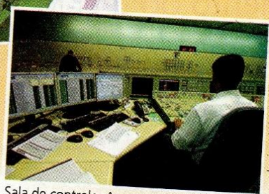
Sala de controle, Angra II, RJ, 2007.
