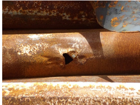
Figure 3.2 – Erosion of pipe from a fluidized bed combustor inbed.
