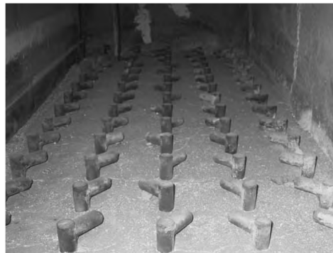
Figure 4.3 – Arrangement of directional nozzle tuyeres.
